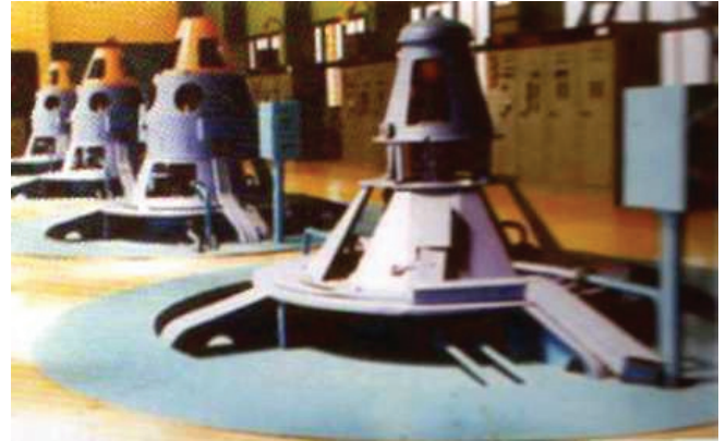
Machinery room at pumping station
