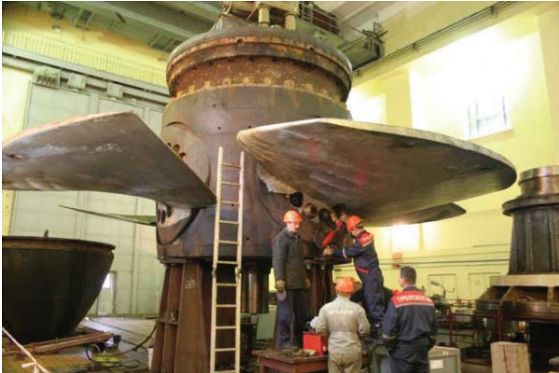
Nizhegorodskaya Hydro Electro Power Station
